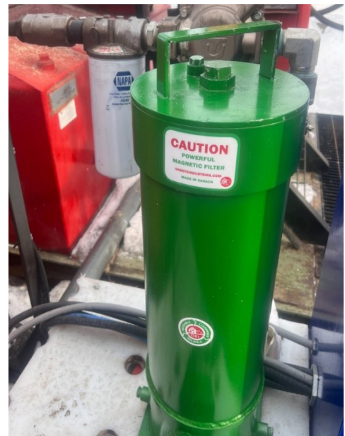
Figure 1: OEI ADD-Vantage 924 series installed on the fuel dispenser.
